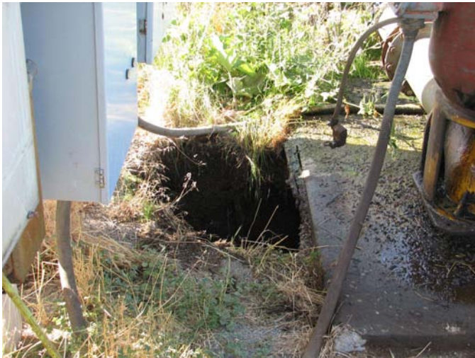
Sink hole 2'x10'x10' the result of a tiny water leak.
