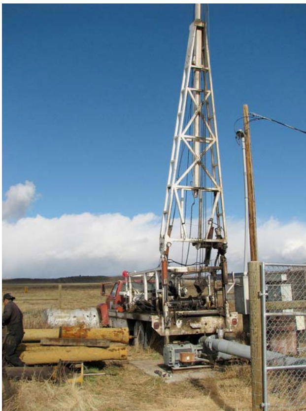
A drilling rig was brought in to hoist the heavy, new pump into place.
